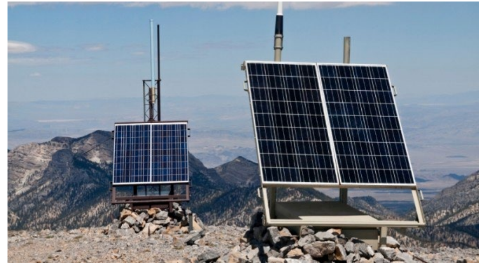
Figure 4: A Solar-Powered Base Station (Source: Google Images)
